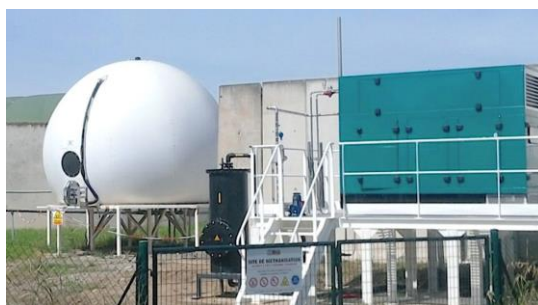
Figure 22. Installation MCube (Source Ovalie Innovation)
